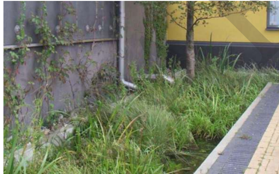
Rain garden catching downpipe water and surfacing run-off
